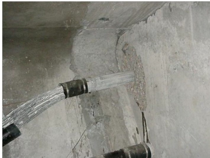
Figure 1.5: Slipping of duct at deviator block ( www.dot.state.oh.us )
