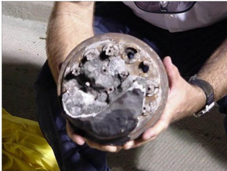
Figure 1.3: Corroded anchorage in Mid Bay Bridge ( www.dot.state.oh.us )
