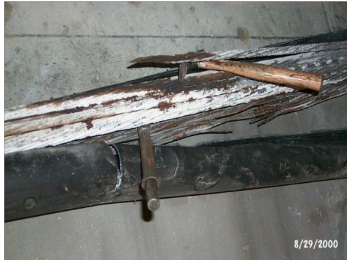
Figure 1.4: Cracked duct showing severely corroded strand ( www.dot.state.oh.us )
